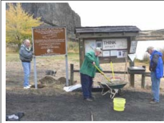
A typical construction project with a worker, a supervisor and a "leaner" L.R.: Pat Kendall, Gary Honeyman and Jerry McBride Photo by Glen Paulson
